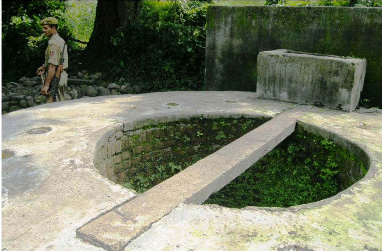
A policeman standing guard near a well that was damaged by upper caste villagers in Rasooh, Jammu and Kashmir. THOMSON REUTERS FOUNDATION/Ashutosh Sharma
